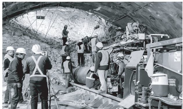
Rescuers in the process of laying a 3-foot-wide pipe through the pile of debris
